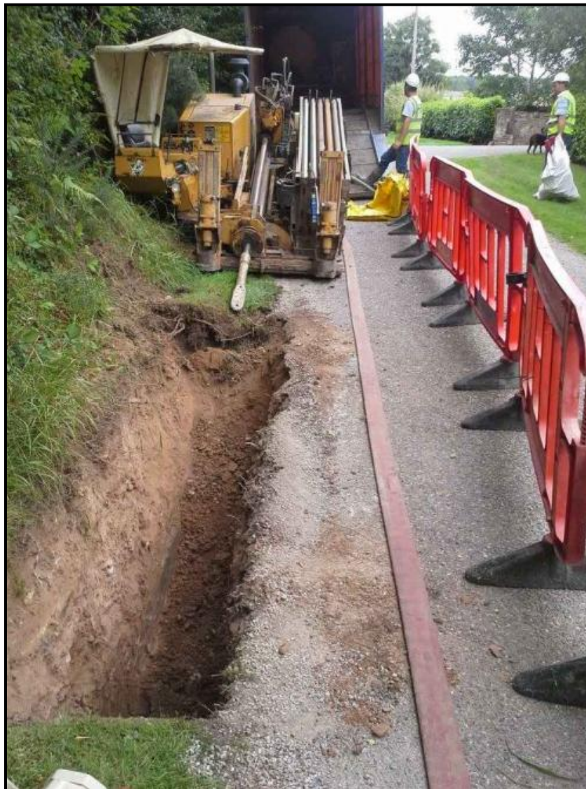
Figure 3-10: Example of a Directional Drilling Launch Pit Adjacent to a Public Road
